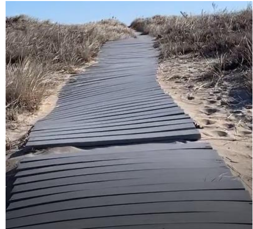
Figure 1: Missing boards; noticeable tilting.
