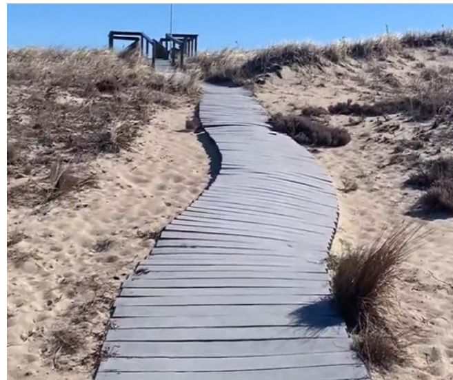
Figure 2: Shifting boardwalk foundation; bare areas of sand and footsteps observed alongside the walkway; Chelmsford Street
