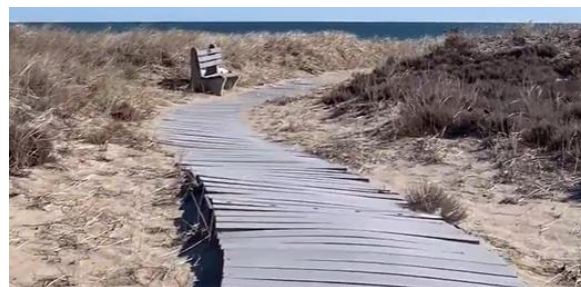
Figure 3: Observed tilting and bowing of some planks; apparent pedestrian use adjacent to the boardwalk.
